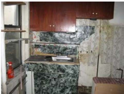
A kitchen in a 60 Hester Street apartment before renovation, with a broken stove and damaged walls.
